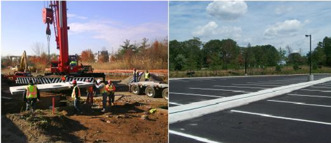
Staten Island's Eltingville Transit Center park-and-ride lot – during construction, and after completion this summer (Source: NYS Department of Transportation).
