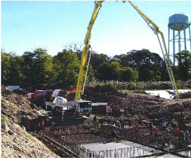
Workers pour concrete for the Village of Greenport's new wastewater treatment facility. (Source: NYS Environmental Facilities Corporation)
